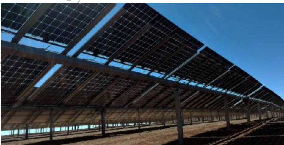
Fig. 2.6 Bifacial Solar PV Panel
