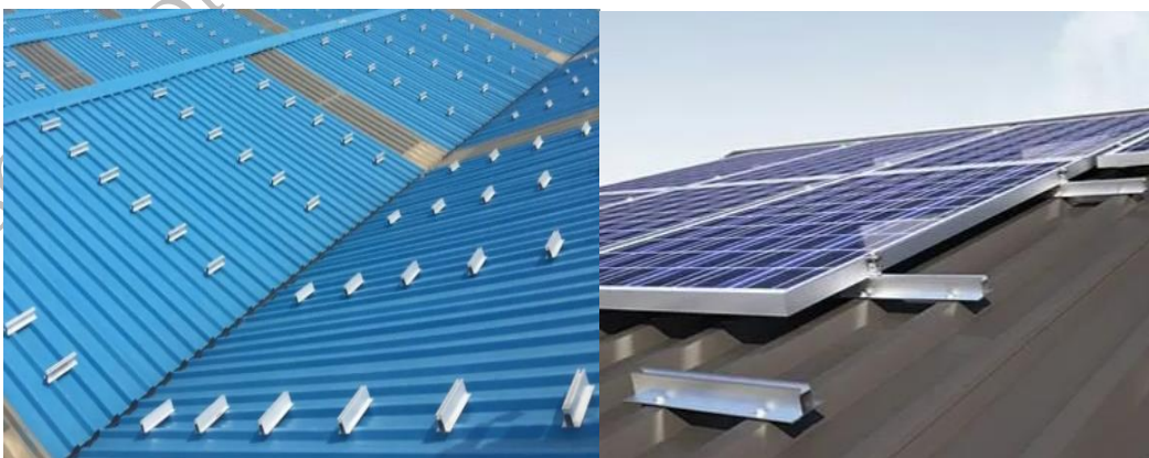
Fig.2.18 Tin Shed Mounting Structur
