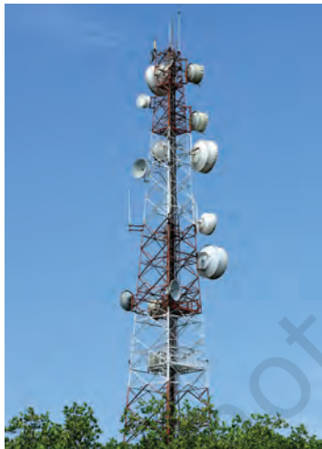
Fig. 2.13: Mobile tower uses microwave for communication
