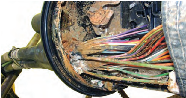
Fig. 5.2: Damage in splice enclosure due to water
