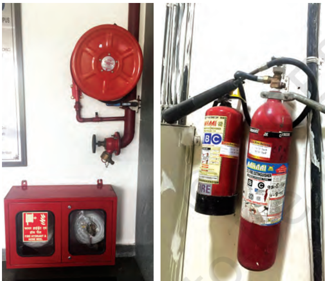
Fig. 5.2(a, b) Fire extinguishers
