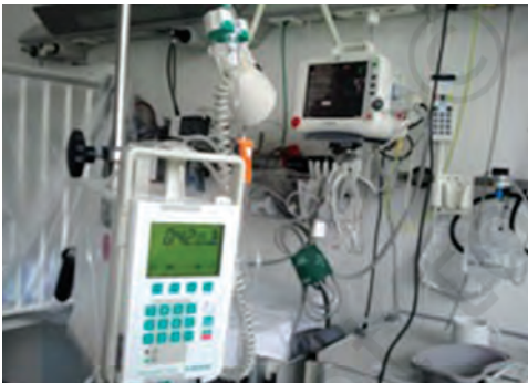
Fig. 5.2 Hospital electrical equipment
