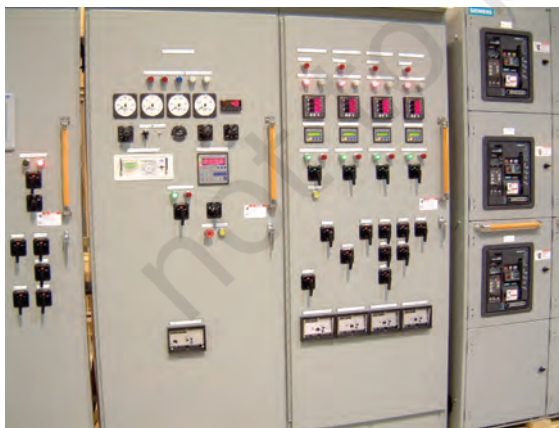
Fig. 8.8 Switch gear cabinet in control panel
