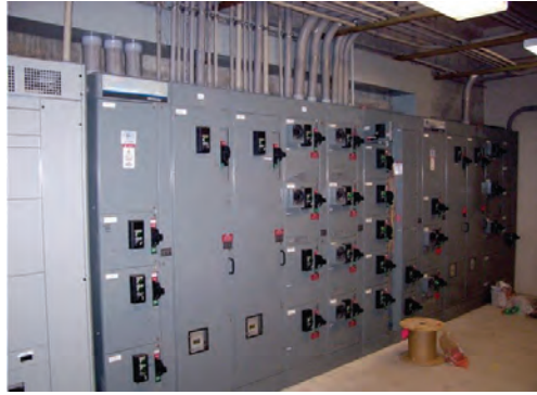
Fig.8.10 Motor control centre in control panel
