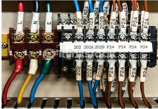
Fig. 8.24 Wires having numbers on the laminated labels
