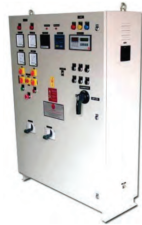
Fig. 8.4 Electrical control panel cabinet
