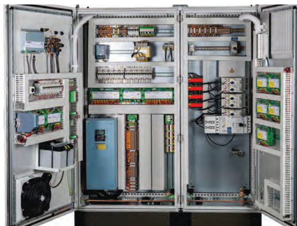
Fig. 8.9 Control cabinet in control panel
