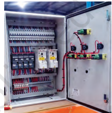
Fig. 8.17 Another way of cabling and wiring
