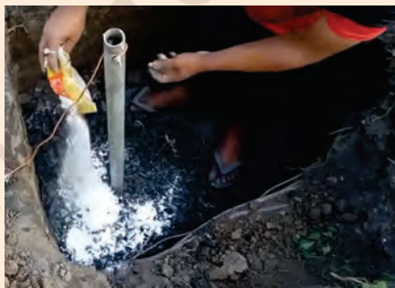
Fig. 3 Copper plate and surface are connected with a pipe
