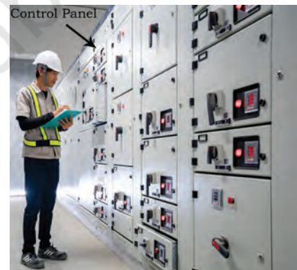
Fig. 1.1(a) A wireman monitoring a control panel
