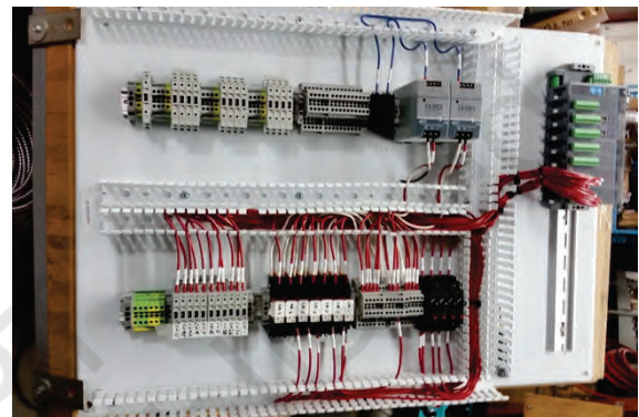
Fig. 8.21 Wireways or cable ways placed on the board
