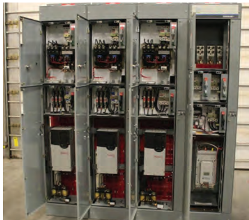
Fig. 8.11 MCC bucket centre assembly in control panel
