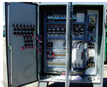
Fig. 8.26 Board inside the panel
