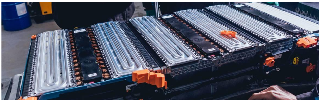
Fig. 5.11: Battery system inspection
