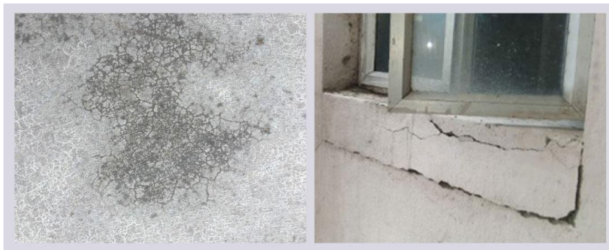
Fig.3.5 Plaster de- Bonding defect
