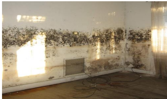
Fig 3.2 Moulds on wall
