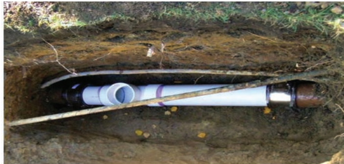
Fig. 4.12 Exposed underground sewer pipe
