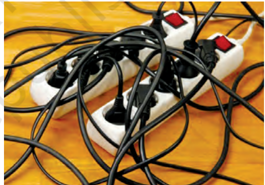
Fig. 1.29: Overloaded extension cords
